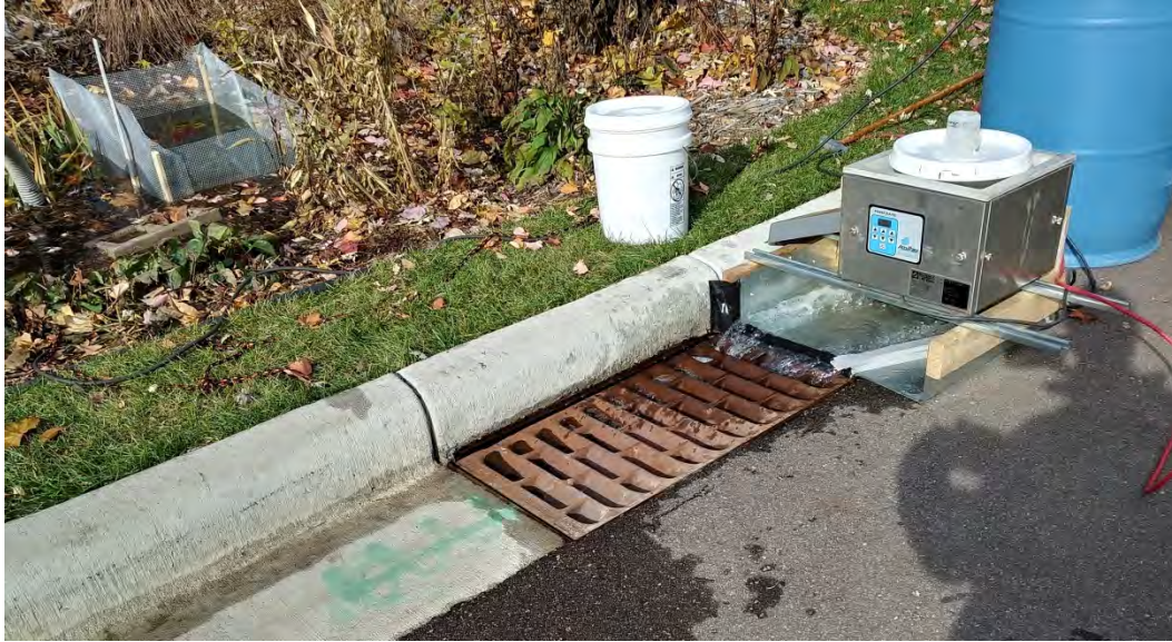
Figure 21. Bloomington field site during pre-wetting flow. Flow enters the shallow sump through the curb grate and emerges into the fenced area of the rain garden through pipes, shown in a subsequent photo.
