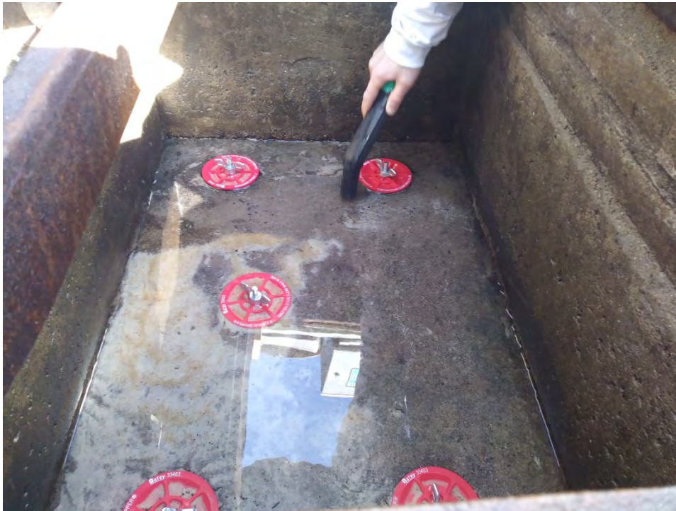
Figure 46. A wet-dry vac was used to remove sediment from the bottom of the Bloomington sump. The red plugs were inserted to seal infiltration holes in the slab to limit sediment loss.
