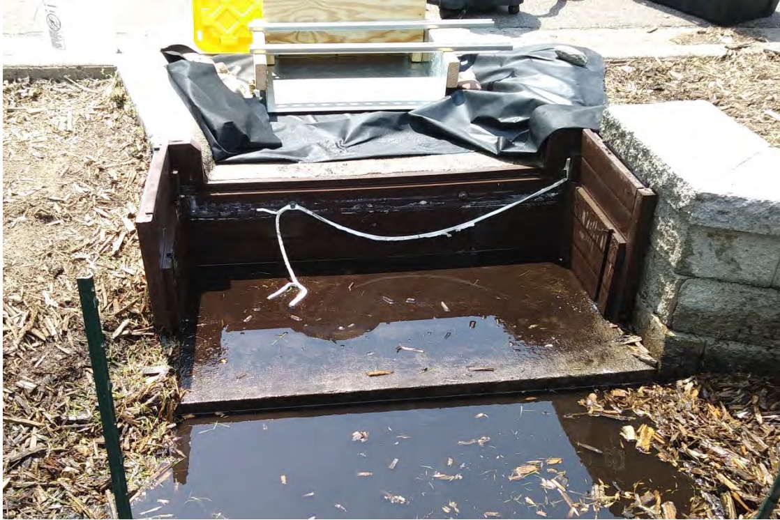
Figure 4. At the Anoka site, the outer frame and concrete pad of the Rain Guardian Bunker device was left in place and adapted for all tests.
