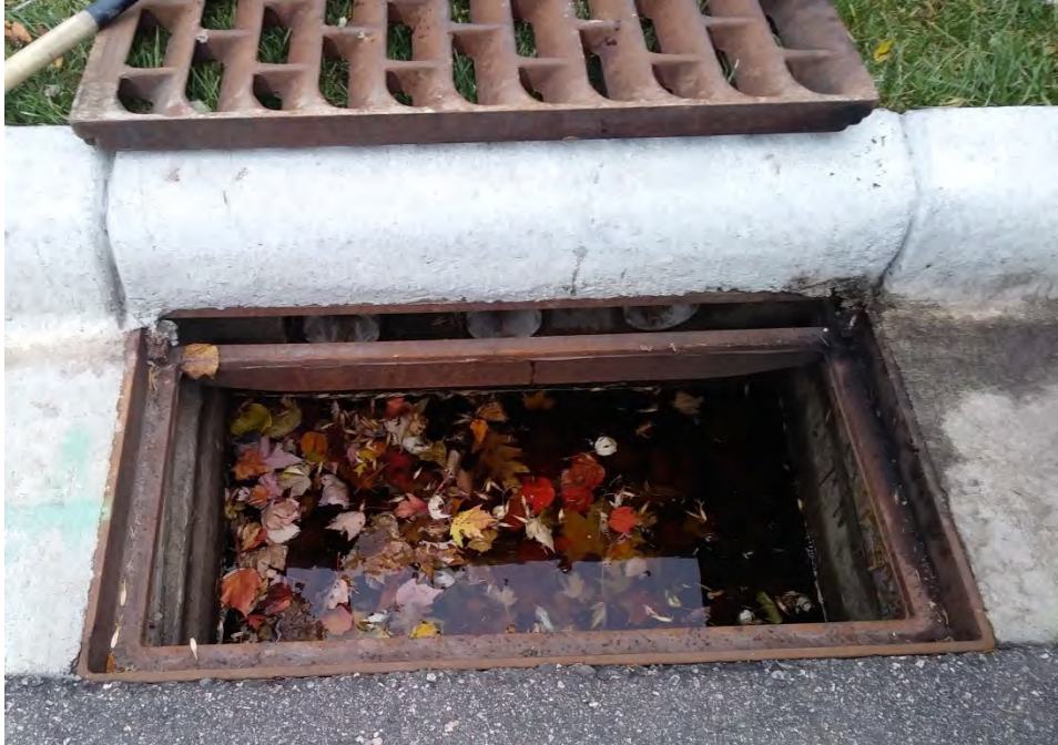
Figure 13. Shallow sump pretreatment with surface grate removed. This photo was taken upon arrival at the site, before cleaning the sump in preparation for testing.
