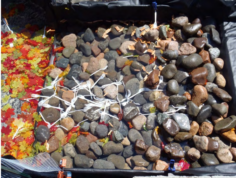
Figure 12. Rock lined inlet after testing at 0.50 cfs for 20 minutes. Entrance from the curb cut comes into the RLI from the right of the picture; exit into the bioretention practice at left.
