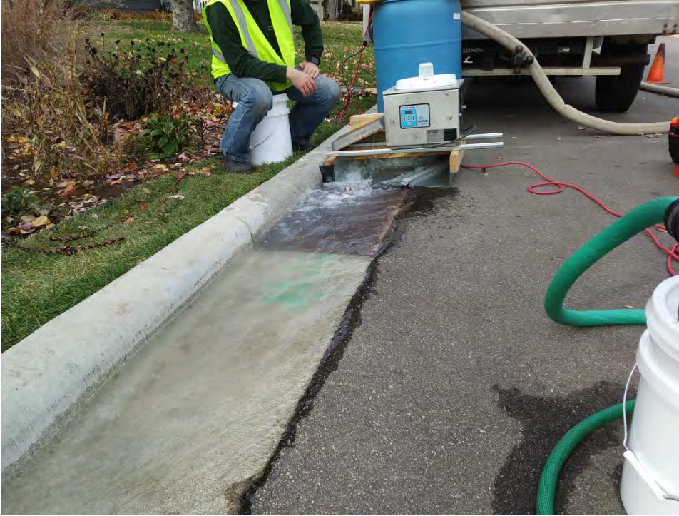
Figure 49. Flow in the gutter during bypass (BBP-025-A).
