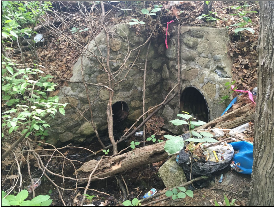
Photo No. 1: View of headwall where intermittent stream discharges from along Thurston Street, facing north toward flags A-8 and A-9.
