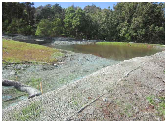
A sediment basin with earthen embankments stabilized with erosion matting and hydroseed.
